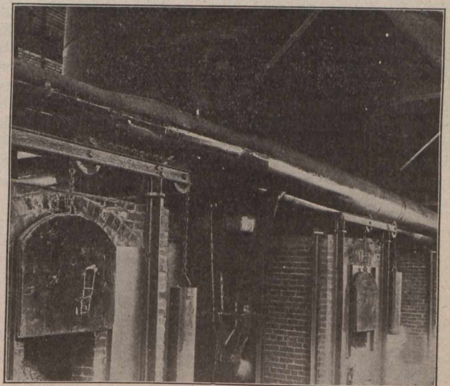
Arrangement of Charging Doors of Kilns.
