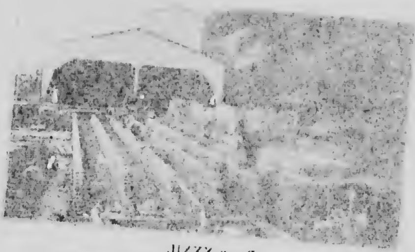
PLATE XXVII. A Digging tunnels under construction at the plant of the Citadel Brick Co. B Setting brick in a scove kiln.
