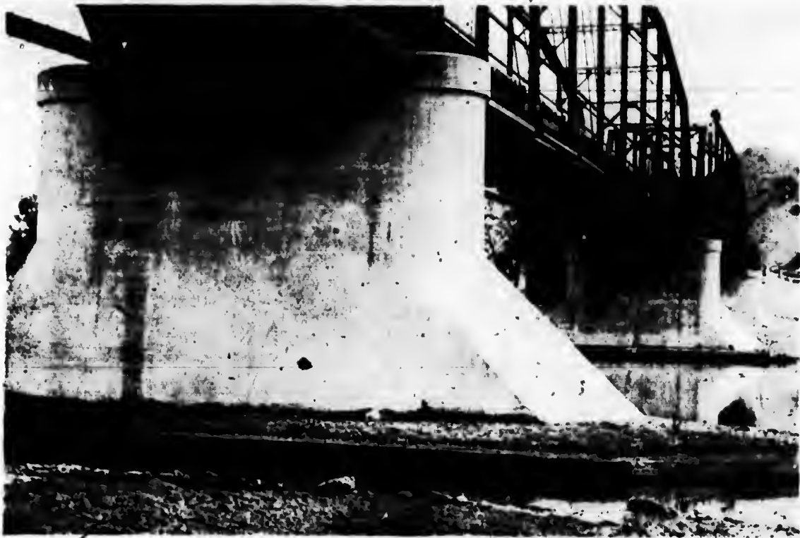
The above illustration shows the very handsome and substantial concrete substructure used for Old Man River Bridge at MacLeod and similar substructure was used for Belly River Bridge, at Lethbridge. The superstructure for these spans (built by us) are shown on pages No. 30 and 31.
