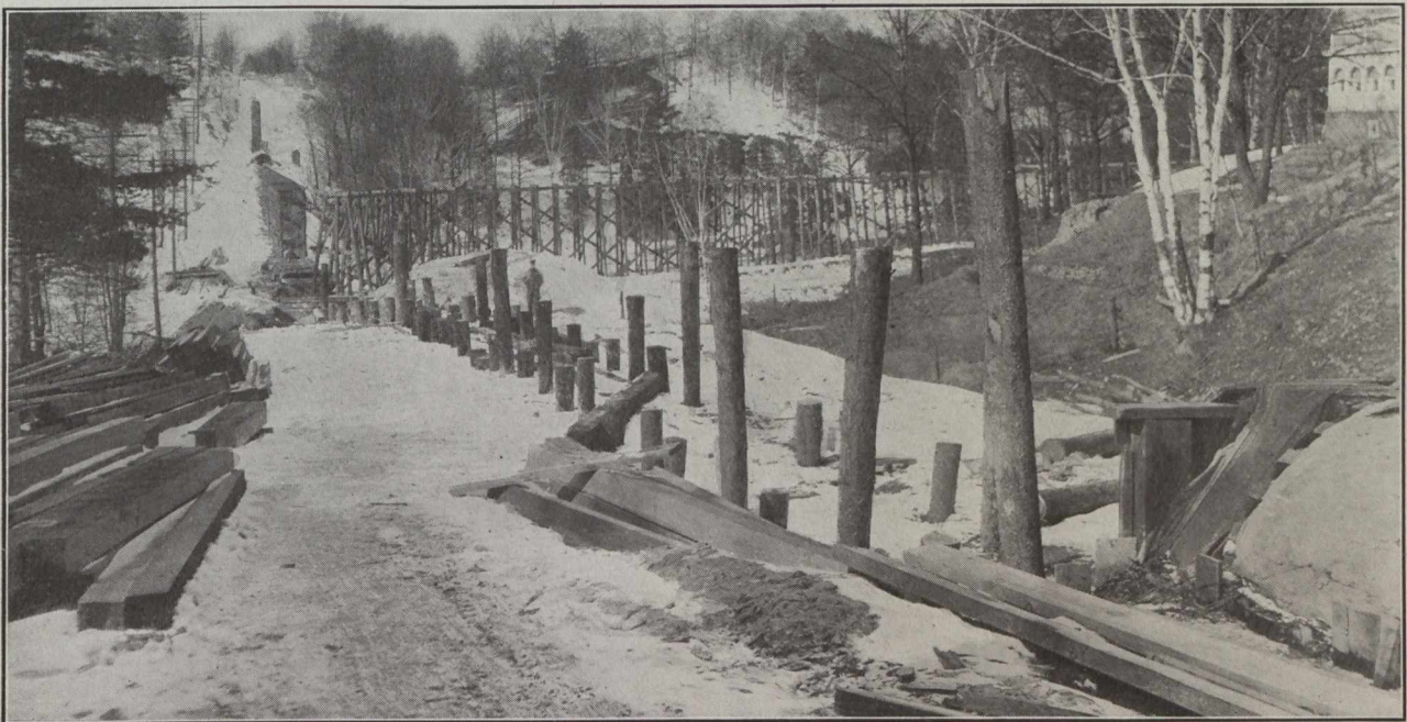
Fig. 1.—Early Construction Operations at Bloor Street and Clendennan Avenue, Showing Piling to Support Timber Trestle to Carry the Bloor Street Line Westward and the Clendennan Avenue Branch Northward.
