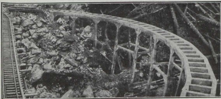
Fig. 2.—Showing Temporary Wooden Railway Trestle and Permanent Concrete Trestle for the Concrete Flow Line.
