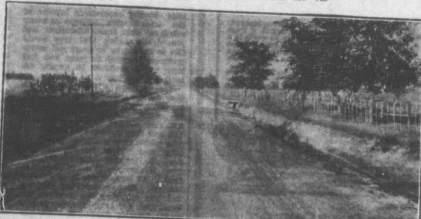
A Clay Road that is Kept Good by Draining. Good roads depend not so much on the material of their construction as upon good drainage and careful maintenance. Note that on this clay road in Essex County, the crown being somewhat excessive, the surface was dragged from the centre outward.
