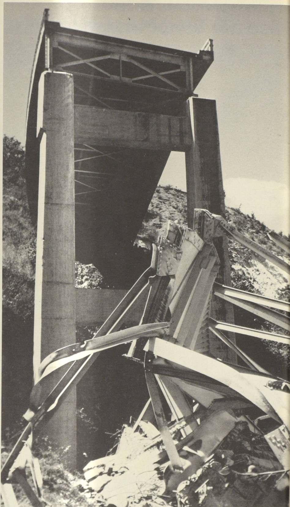
Dr. D. H. Weichert , Division of Seismology and Geothermal Studies, Energy, Mines and Resources Canada, went to Guatemala following the devastating earthquake there last year. His photograph shows a fallen span of modern highway bridge across Rio Platanos, interrupting CA9, Guatemala City's main supply route from the Atlantic coast.
