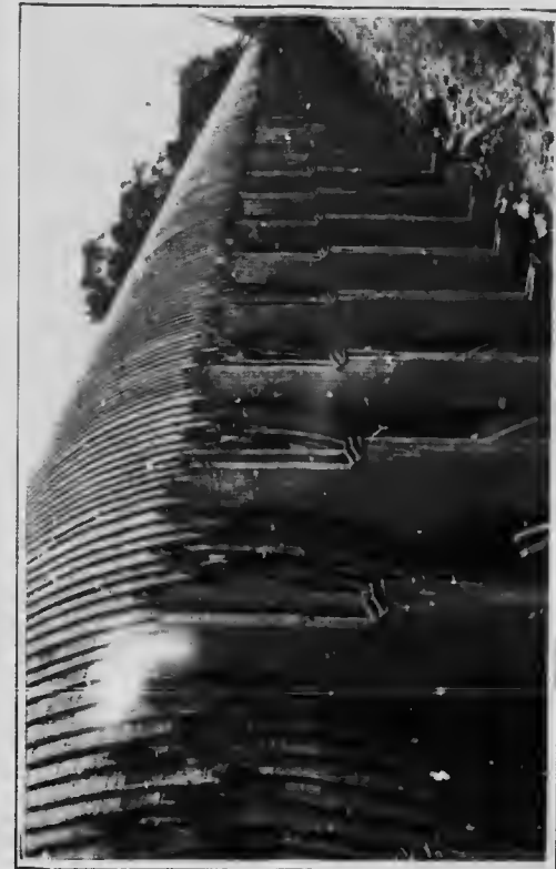
Wood stave pipe, showing details of bands, shoes and saddles
