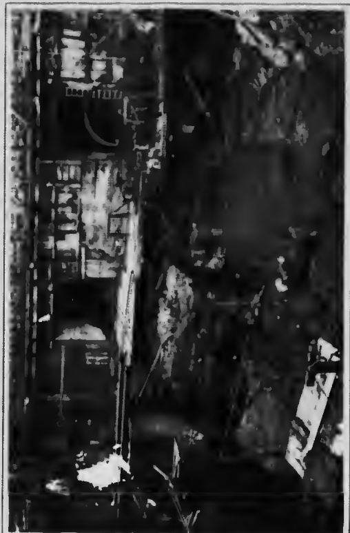
Power house extension site ready for forms. Two tunnel portals appear in background with posts, & No. 40 being assembled. Draft tube form for No. 18 in position
