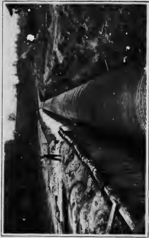
No. 3 conduit completed, showing method of bracing Lackawanna steel sheet piling between conduits Nos. 2 and 3
