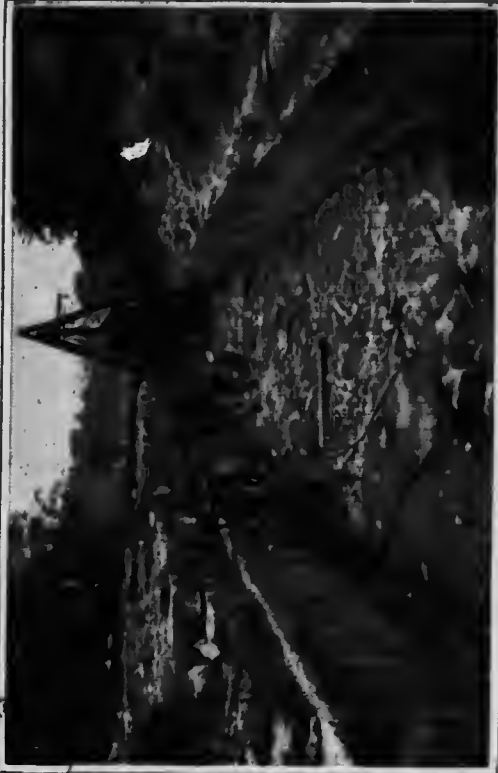
Rock excavation in pipe trench near International Railway crossing. Rock drills at work
