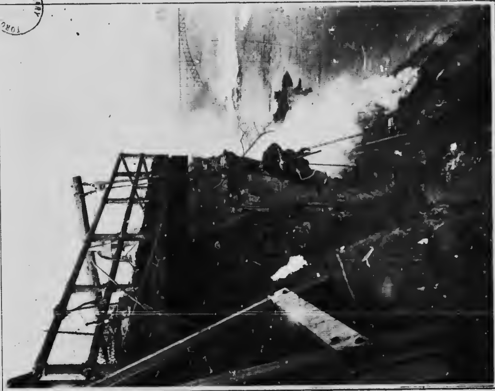
Scaling loose material from cliff above power house site. International arch bridge in background
