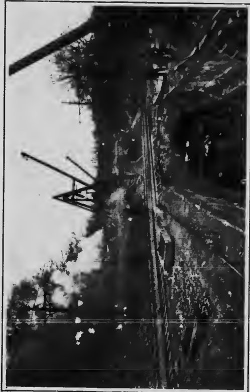
Trench for wood stave pipe through rock section, showing tunnel beneath International Railway Company's tracks. Both sides of cut are channelled here
