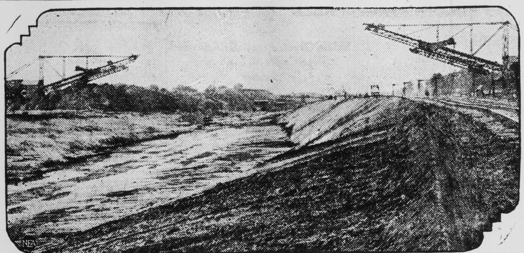
Here is a comprehensive view of a section of the River Shannon Power Canal at the Black Water end. Near here is to be located the dam which indirectly will provide the 50,000 electrical horsepower.
