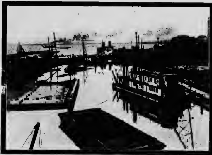
CONSTRUCTING THE ENTRANCE FROM TORONTO HARBOR TO THE NORTH SLIP, INDUSTRIAL DISTRICT.
