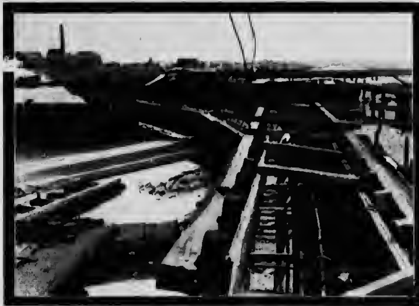
BULKHEADS READY TO RECEIVE CONCRETE ON LAST FURCE OF CONCRETE WALL, NORTH SLIP.
