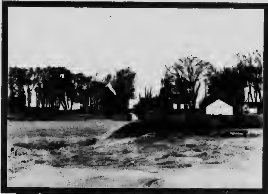
THE DISCHARGE FROM A HYDRAULIC DREDGE—PUMPING SAND AT THE RATE OF 1,000 CUBIC YARDS PER HOUR.
