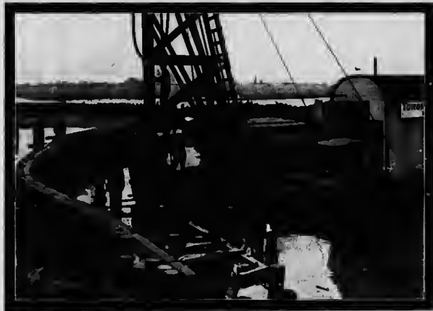
TEMPORARY BULKHEADS BEING PLACED TO DIRECT THE 17,445,000 CUBIC YARDS OF SAND BEING PUMPED INTO THE DISTRICT.
