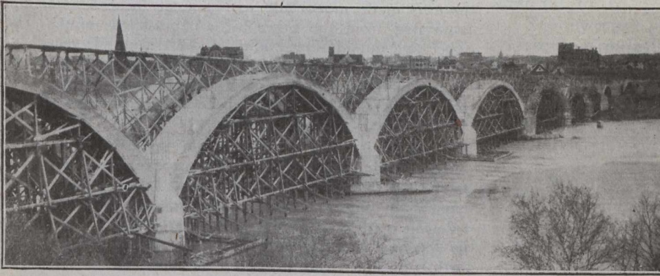
Showing Timber Centering for Arches Carried Upon Piles, Trestle Carrying Concrete Delivery Pipe, and Reinforcing for Spandrel Columns.
