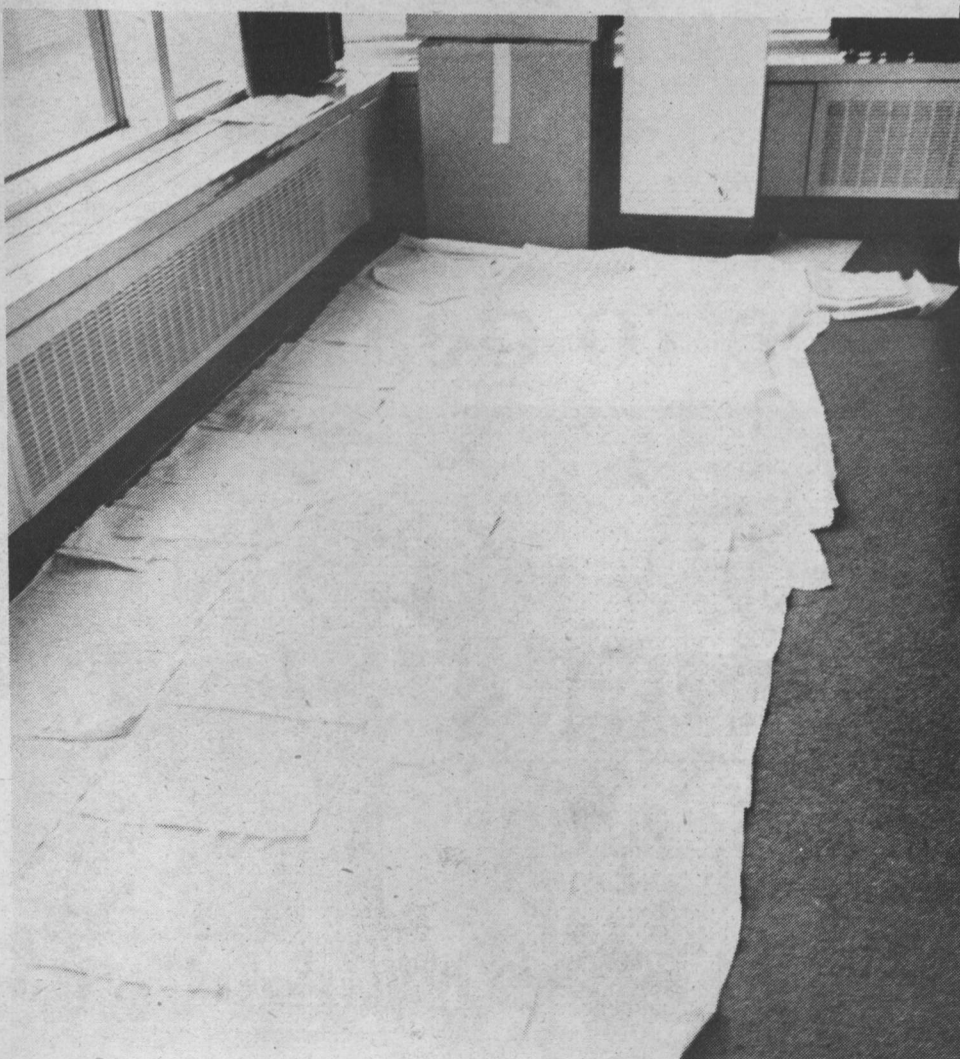
A vandal-instigated flood in the SUB tower caused irreparable water damage.
