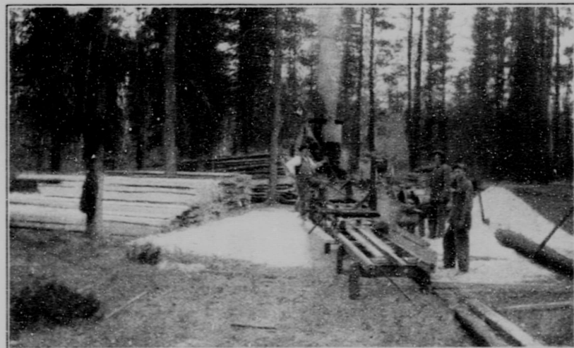
Reducing the Cost of Building. Settlers in Central British Columbia Cutting Their Own Lumber.
