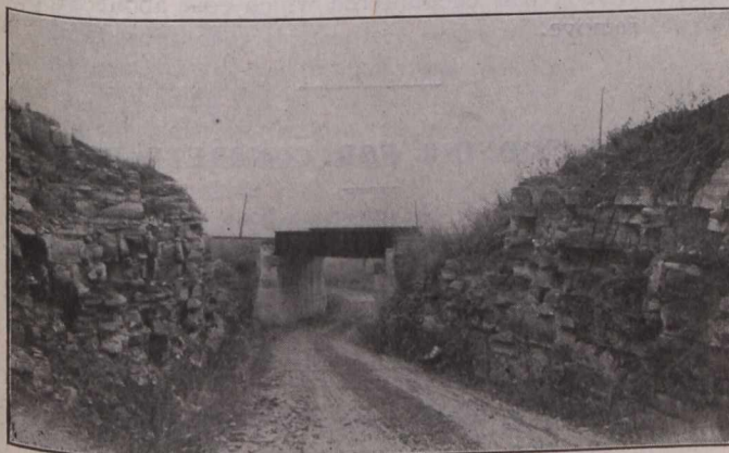
A Dangerous Subway
