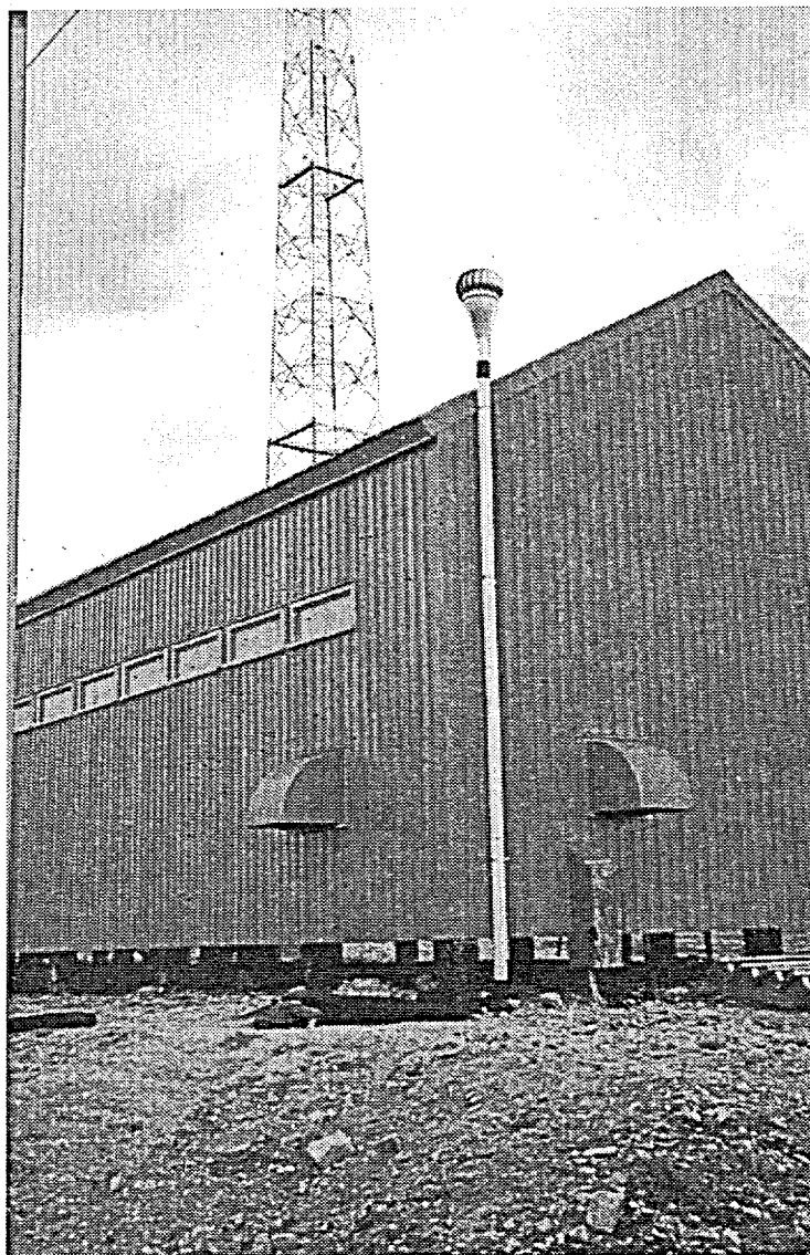
Figure 4. View to southeast showing vapour extraction exhaust stack attached to the side of the transmitter building. The turbine is visible at top of pipe.
