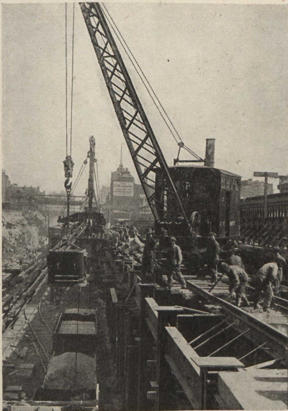
Digging out the Solid Rock and Building the Two Decks of Tracks which carry New York Central Trains in and out of the heart of Manhattan.
