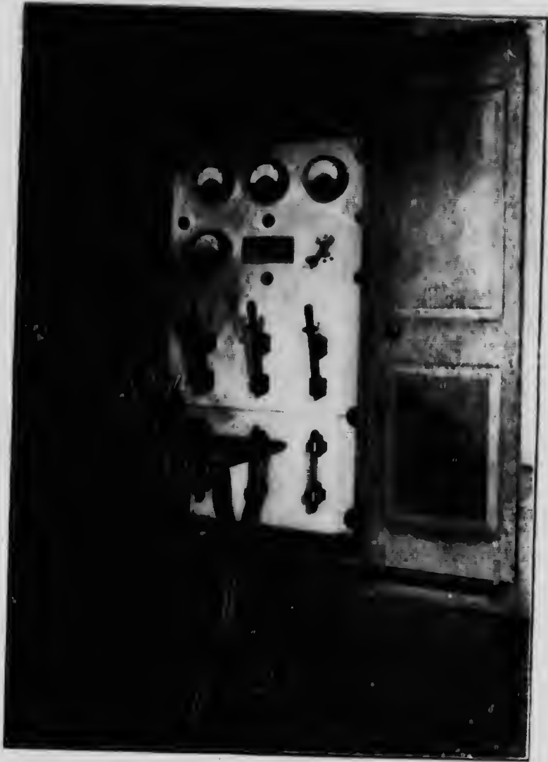
General View of Switchboard and Valve Stand for the Stassano Furnace.
