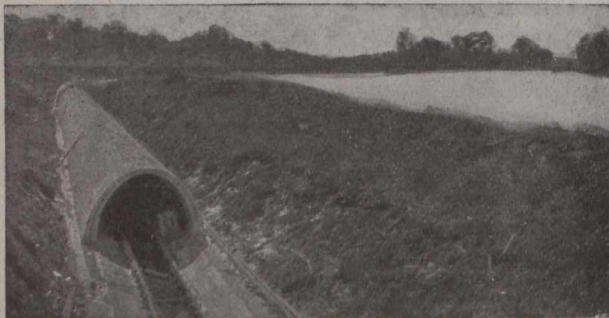
Completed Aqueduct Before Backfilling. View along the shore of Indian Bay. The intake is just over the rock ridge in the middle centre. The dike is holding out about 3½ feet of water that would otherwise float the surface.
