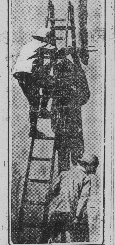
Picture of Italian soldiers installing telephones in Tripoli. The Italians hold the city fort, but the outer forts are in the hands of the Turks. TRIPOLI. - One of the first things the Italians did on capturing Tripoli was to install telephones in the city, and if it were not for the serious side, for now this city is again besieged from the land side by Arabs and Turks, one could smile at the incongruity of the placing of what represents the new age in buildings that are almost as old as the hills.
