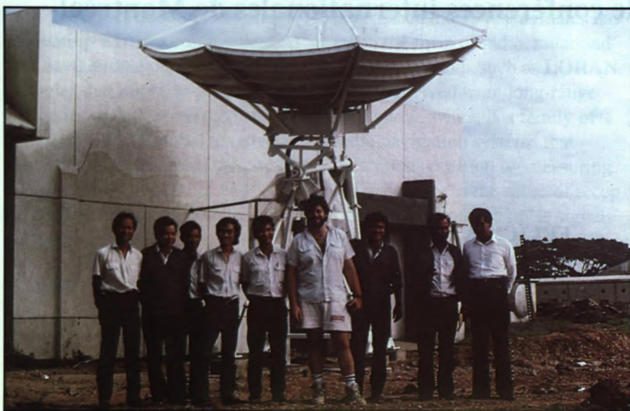
Canadian expertise in satellite communications is being provided in Vietnam where Calian Communications Systems Ltd., formerly Skywave Electronics, has furnished and installed a two-node network for more effective air traffic control.
