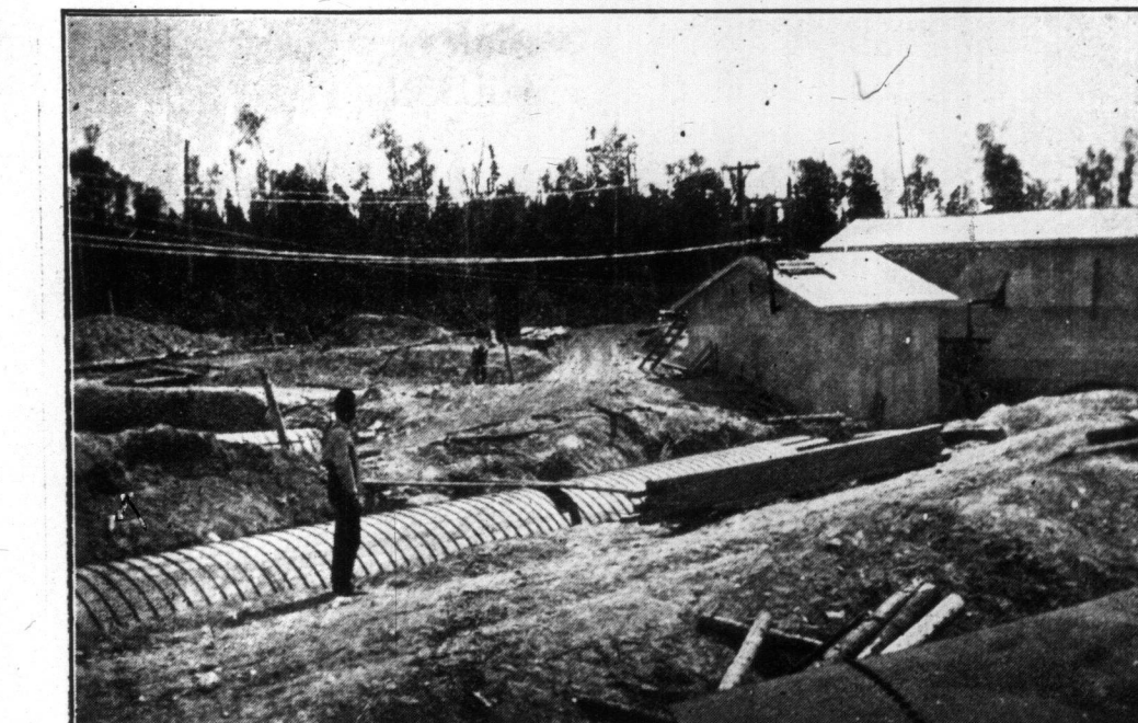
Housing Over Valve on Wooden Stave Pipe, and Over Intake at Canal Entrance, Wawaiten.
