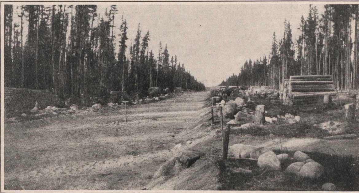
Between Dufferin City and Pine City—Specimen of a new road chopped and built along the line of one of the new railways in Northern Ontario.
