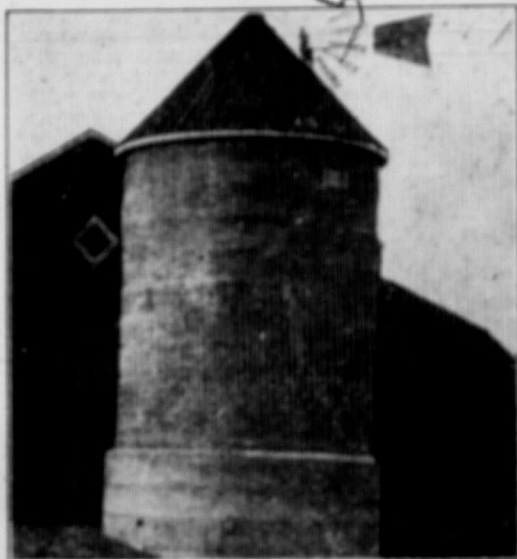
Solid concrete silo on J. D. Turner's farm, Carroll, Man. Solid concrete is solid and durable but breaks rather badly. This one is partly underground, making that part like a 'pit' silo.
