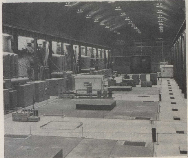
Outardes 3, completed in 1969, is an underground power-house.
