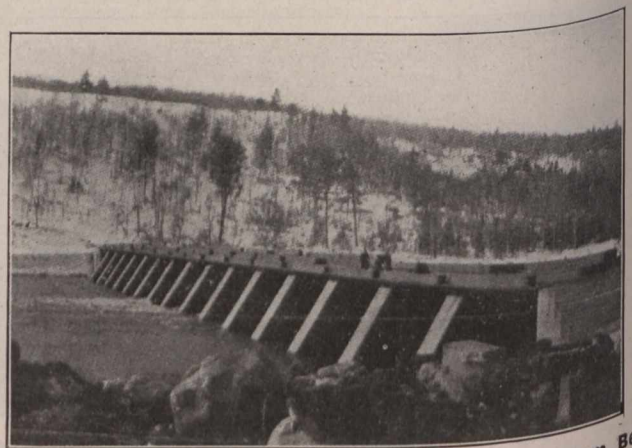
Fig. 3.—Timiskaming Dam. Ontario Sluiceways from Below, Showing Water on Lower Apron and Stop-Logs Piled on Roadway.
