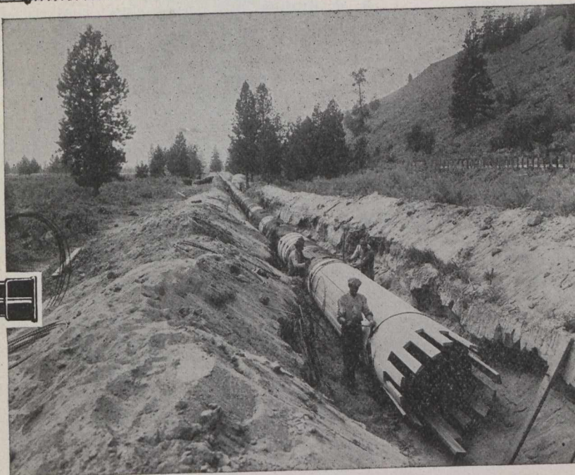
48 in. CONTINUOUS STAVE LINE.
