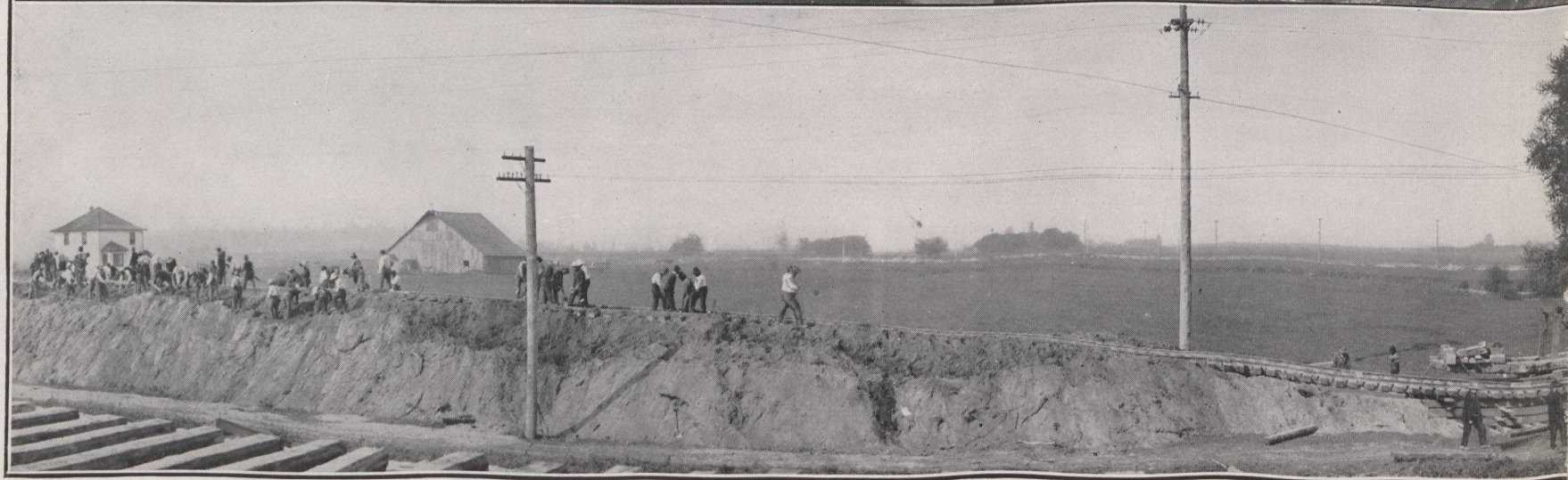
BUILDING THE EXTENSIVE TRANSCONTINENTAL CANAL Locomotives, Donkey Engines, Work Trains, Ditchers, Dredges, and Hundreds of Horses and Men have Tilled on them for Months—Second Division of
