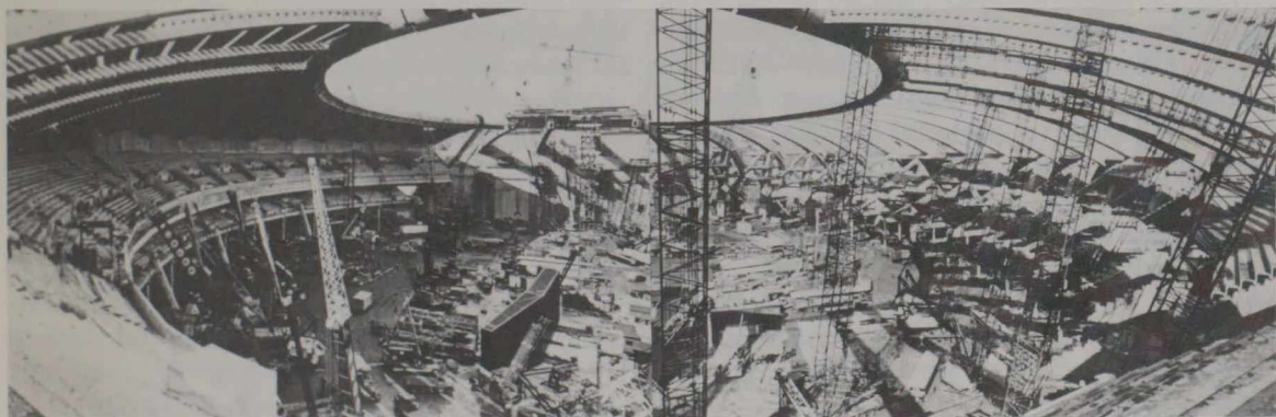
Top: The uniquely splendid stadium complex in April as it entered the last stages of construction. Bottom: The Stadium in March.
