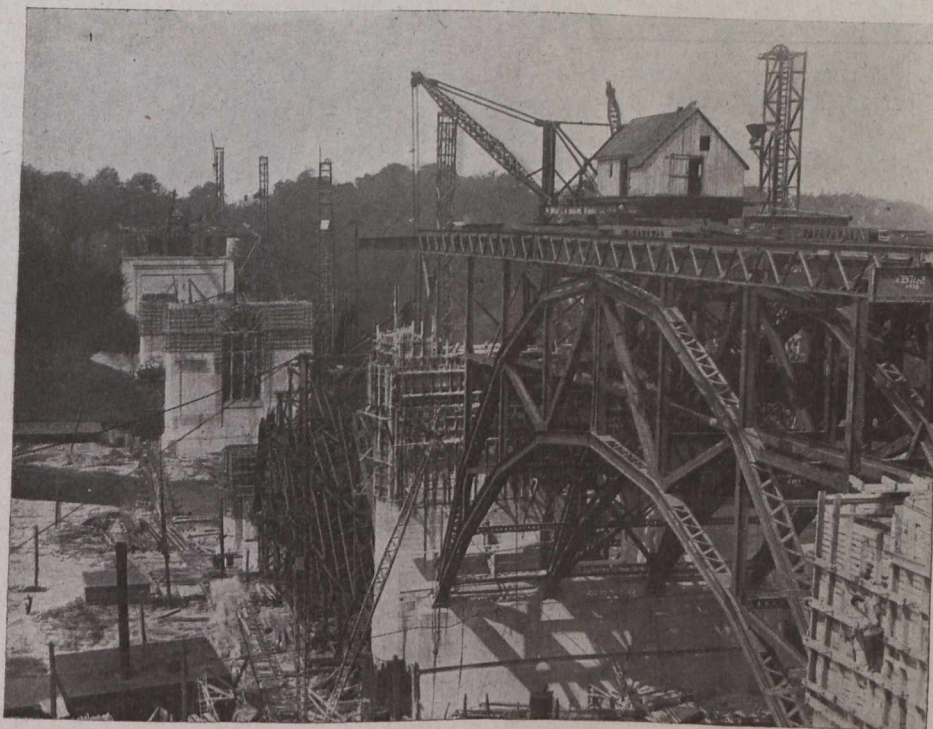
Fig. 1.—Don Section, Bloor Street Viaduct, Looking West from Pier A (near Danforth Avenue). Photo July 27th, 1916.
