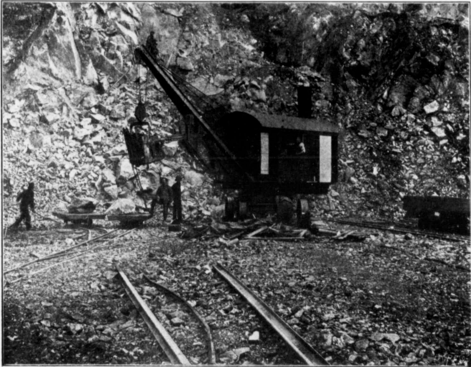
Steam Shovel at work in No. 1 Pit—Mouth of Tunnel hidden by loose rock.
