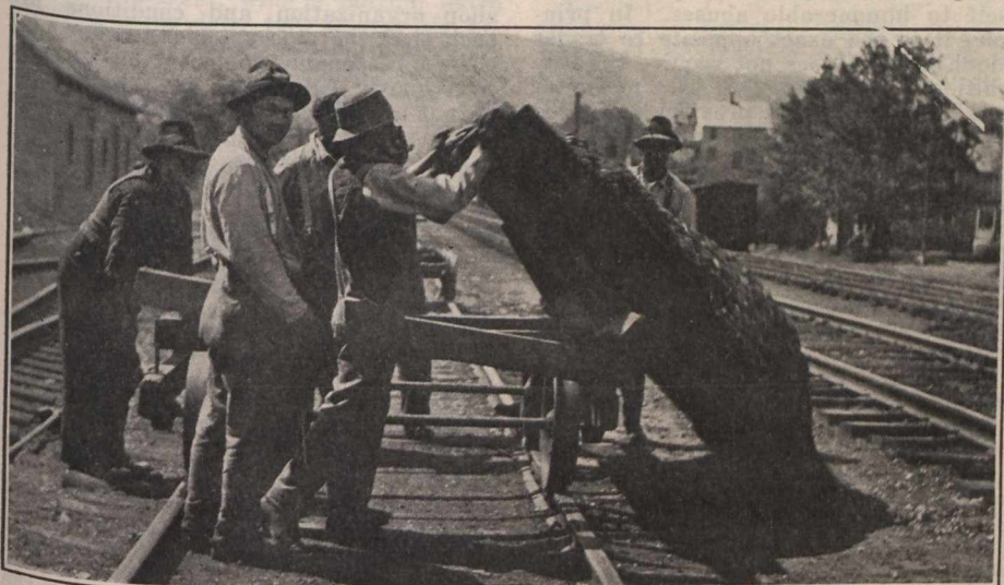
Push car, dump box being emptied. Material may be spread by moving car as load is released.
