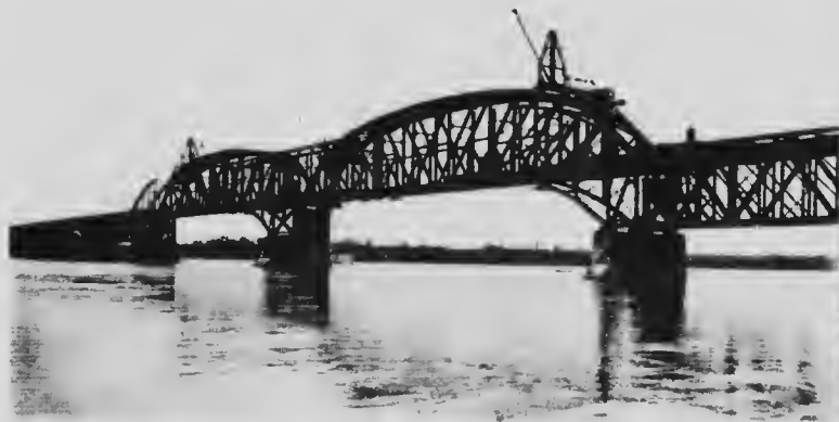
1st and 2nd 498 foot spans ready to launch Dismantling old channel spans
