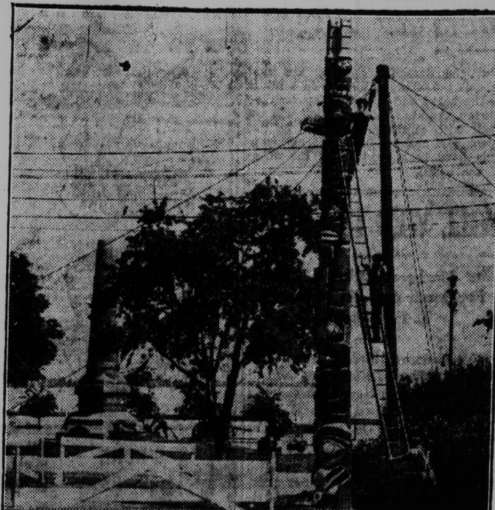
A British Columbia totem pole being erected in an historic corner of the Canadian National Exhibition grounds at Toronto, just beside the monument which marks the site of Fort Rouille, the first white dwelling place in Upper Canada.
