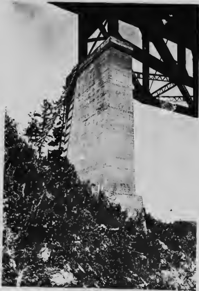
Single pier of Bridge on St. Maurice Railroad, Shawinigan Falls P.Q. International Portland Cement used.
