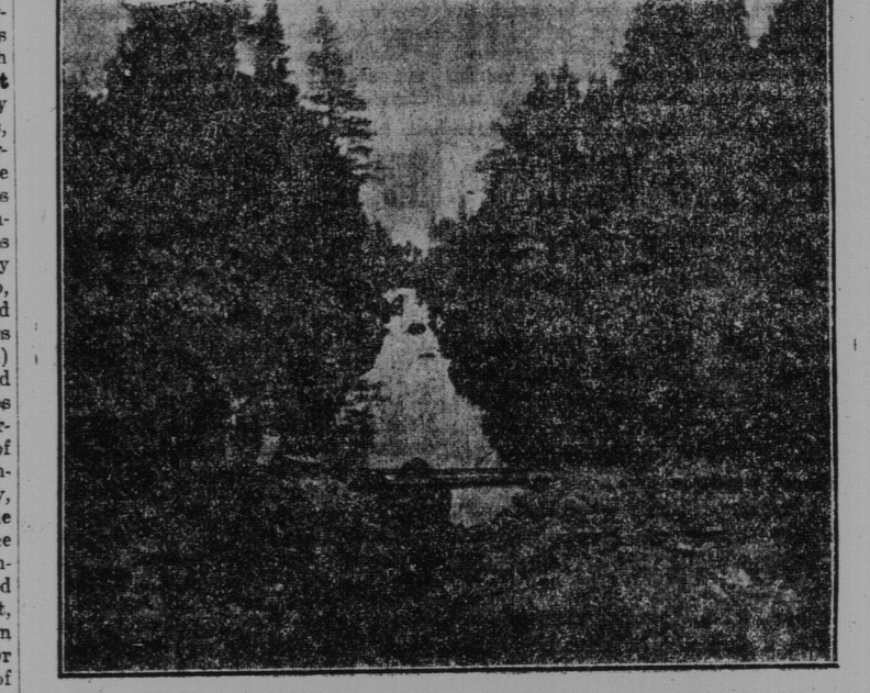
Looking Down the Pipe Line--Part of Rock Section Already Blasted and the log sluice which will be near the right bank, the water is being pumped from inside the coffer dam by means of a powerful centrifugal pump. At the time the picture was taken the pump was at work, and the stream of water discharged into the lake. The trellis work bridge in the back
