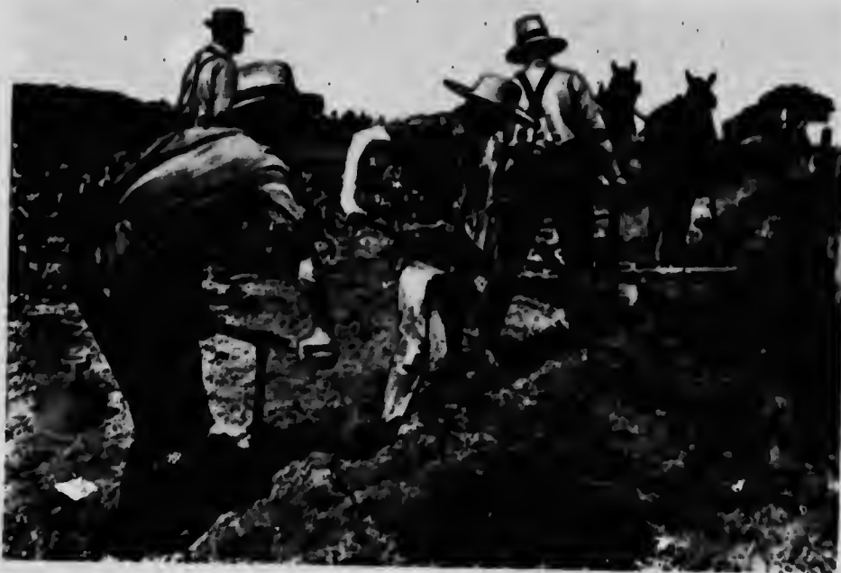
FIG. 11.—Making a trench in western Ontario, showing three necessary essentials, namely, ploughing, deepening and trimming the furrow with spade, and digging post hole. (Photo by J. Moore).
