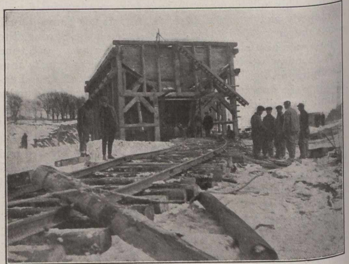
Fig. 2.—Starting Down the Incline. The Track Shown is a Siding from the Construction Railway.
