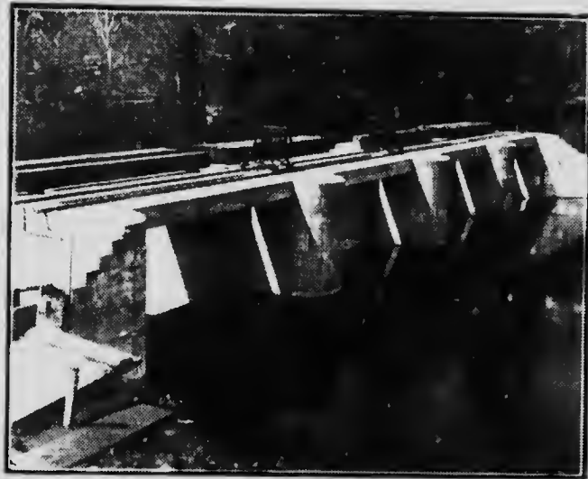
HORSESHOE LAKE DAM ON GULL RIVER THIS IS ONE OF THE RESERVOIR DAMS ON THE TRENT CANAL WATERSHED
