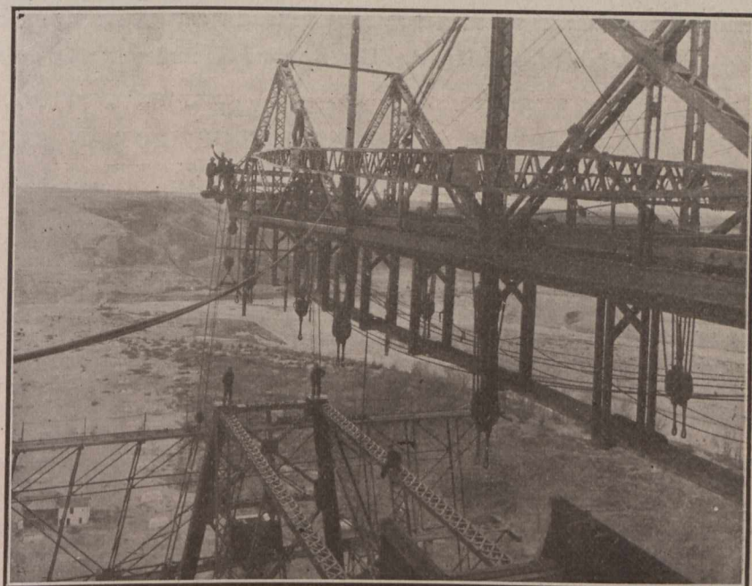
Fig. 21.—Cantilever Arm of Traveller. Note the erection cage suspended at the top of the tower.
