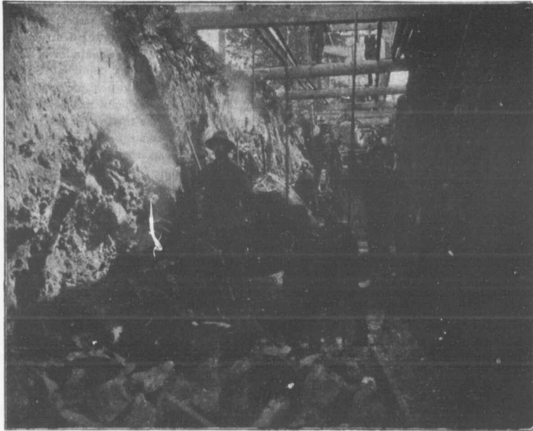
Three out of the ten or our "Ingersoll" steam drills used by Messrs. Laurin and Leitch in excavating rock at St. Louis de Mile End, Quebec. These rock drills are fully described in catalogue No. 87
