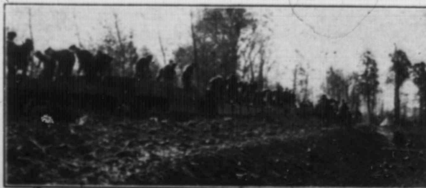
Rapid Railway Construction in France. Broad Gauge Railway being constructed. Building an Embankment.
