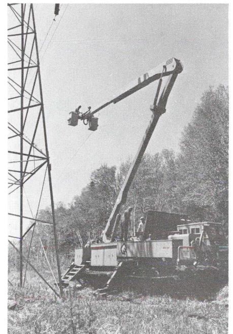
Photo Ontario Hydro
