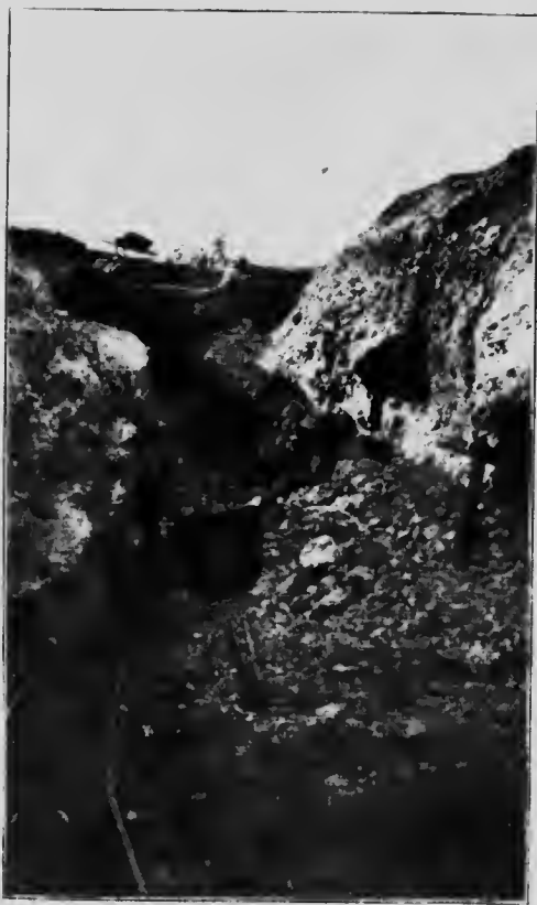
Loading ore at the face in open cut. Lone Star mine, Victoria gulch.
