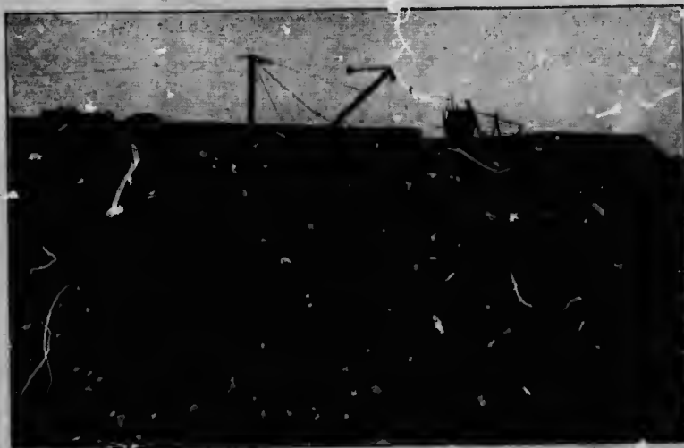
FIG. 10. VIEW SHOWING MASONRY OF REGULATING WEIR AND RACEWAY BRIDGE AT LOCK NO. 4; SOULANGES CANAL WORKS, CANADA.
