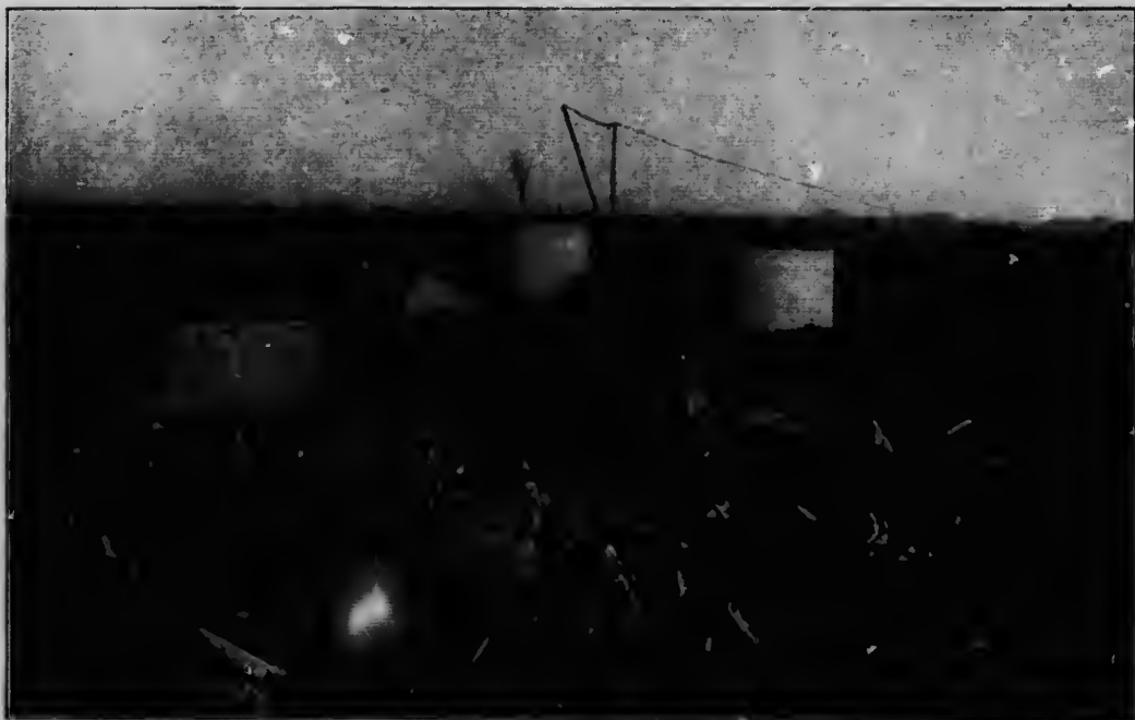
FIG. 12. VIEW SHOWING EARTH SLIP ON SUMMIT LEVEL; SOULANGES CANAL WORKS, CANADA.
