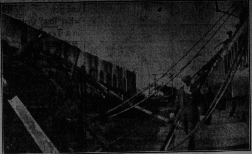
Above depicts the mass of steel and twisted iron which collapsed Tuesday afternoon, smashing down upon train about to depart. The above was photographed by William Noble immediately after the mishap.
