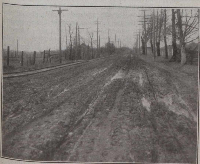
On the Route of the Toronto-Hamilton Highway Near New Toronto. Photo in May, 1917. The farmers along this road will be glad to see the concrete mixers
