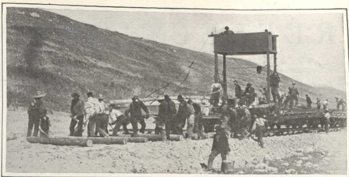
Track-laying machine that lays a mile and a half of steel, including ties, in a day.
