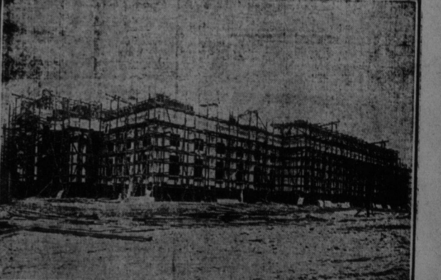
This picture shows the present stage of progress on the magnificent $300,000 pavilion that is being erected by the Dominion of Canada at the Panama-Pacific International Exposition at San Francisco in 1915. The pavilion, as shown by the photograph, is almost structurally complete and needs only ornamentation.
