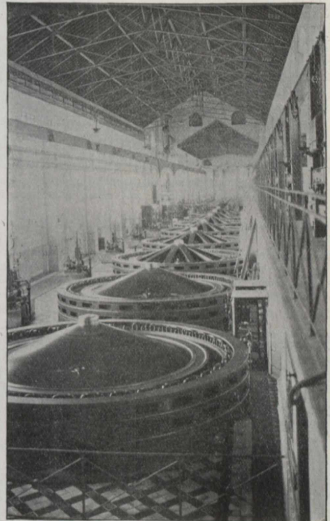
Fig. 2.—Lyons.—Interior of Generating Station on the Rhone.
