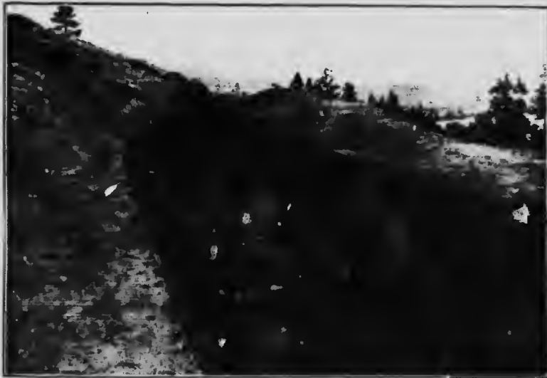
Fig. 28.—Earth canal ready for concrete lining, Fruitlands Irrigation System, Kamloops, B. C.
