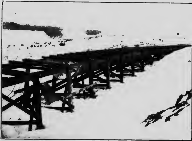
Fig. 35.—Steel flume in process of construction, Fruitlands Irrigation and Power Co., Kamloops, B. C.
