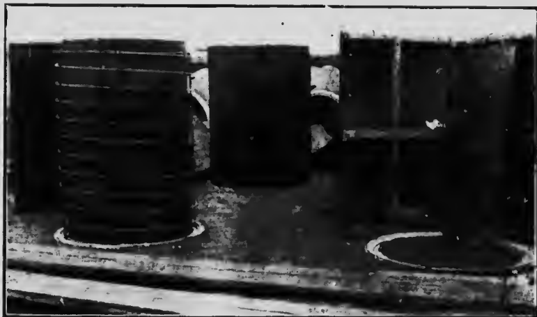
Fig. 12.—Inside core and spiral reinforcement in position for casting 30-inch reinforced concrete pipe, Umatilla Project, Oregon.
