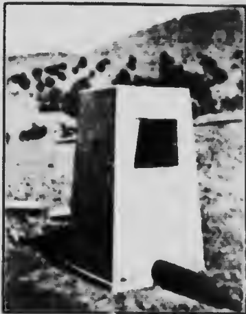
Fig. 12.—Weir box take out valve.
