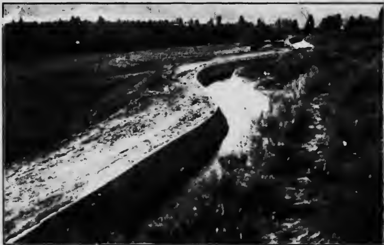
Fig. 24.—Concrete lined canal of Fruitlands Irrigation and Power Company, Kumloops, H. C.
