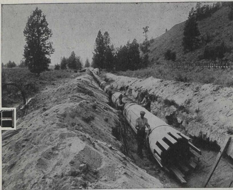
48 in. CONTINUOUS STAVE LINE.
