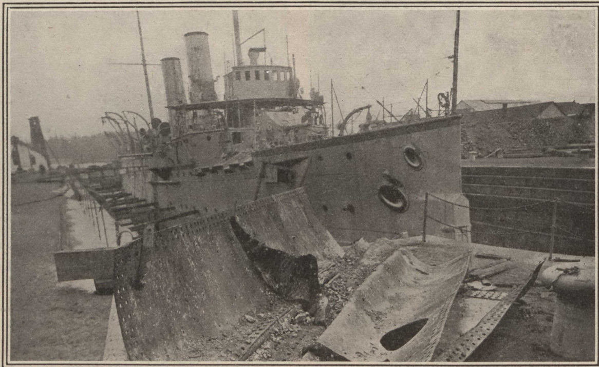
H.M.S. Flora in Dry Dock at Esquimault, being repaired. Torn and crumpled Plates in foreground.
